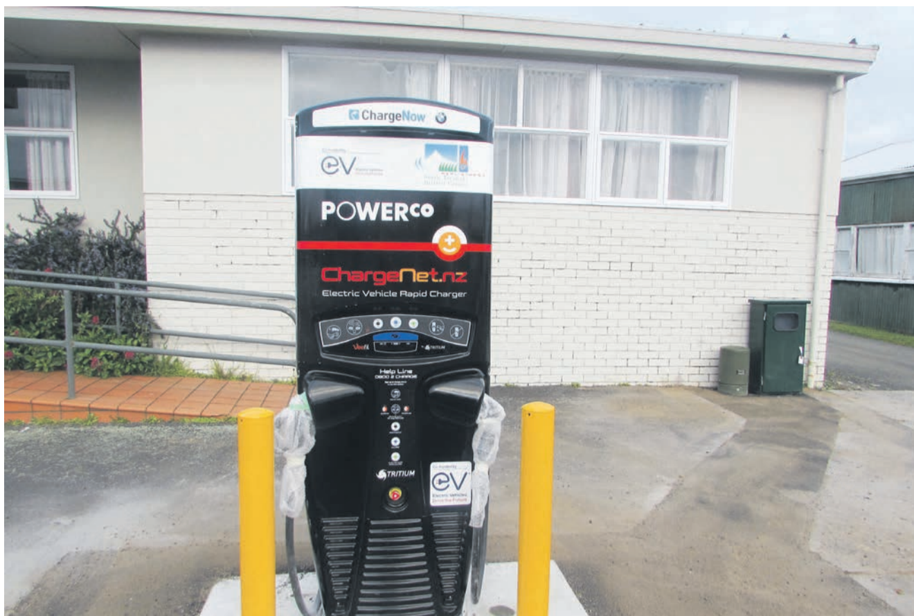
Opunake's new electric charging station.
